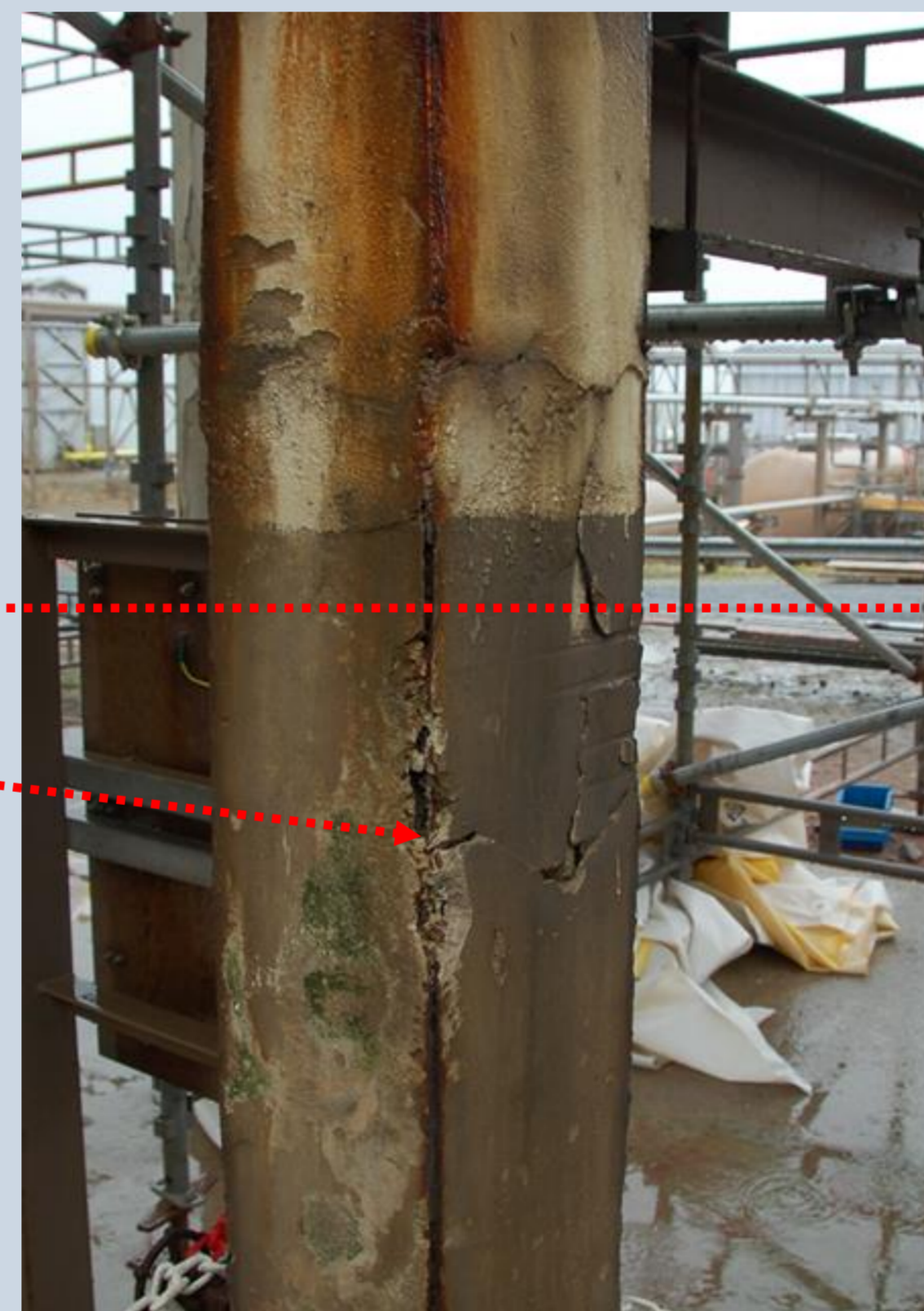
Figure 5 shows typical anomalies; the corner angle bead has corroded, the coating is detached and mechanical damage has compromised the arrangement.
