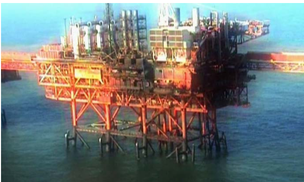
Above: Damaged oil rig – a scene from 'Incredible – The story of Rough 47/3B'
