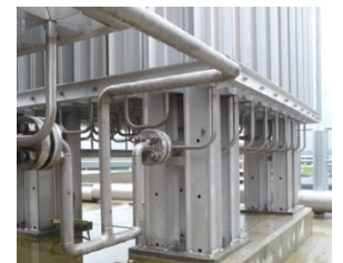
Figure 3: Pipework detail into base of liquid nitrogen vaporisers
